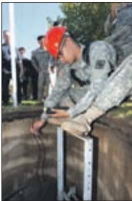
[Left] Spc. Vashaan Johnson is lowered into a manhole on Patch Barracks during Confined Space Entry Training Sept. 23. [Above] Pvt. Angel Diaz uses special equipment to check oxygen levels and ensure that no toxic gas is inside the manhole before being lowered into it.
